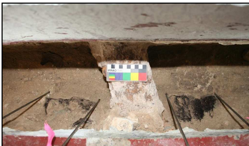
Figure 4. Timber joists in west wall underlying concrete veranda No. 12 The Terrace from above
