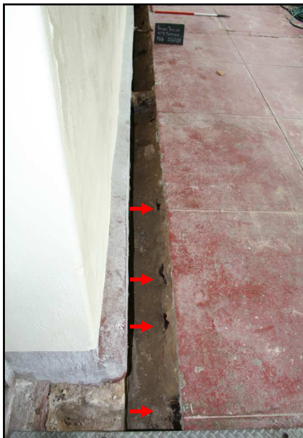
Figure 3. Timber joists in west wall underlying concrete veranda No. 12 The Terrace, looking south
