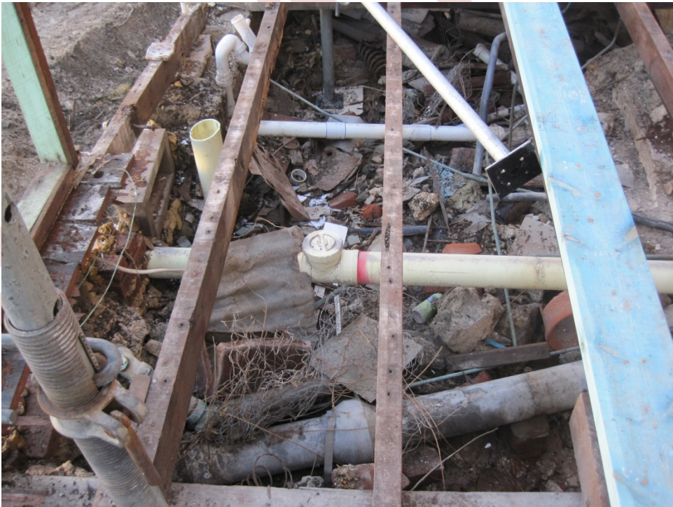
Figure 3 – P877 Warders' Cottages – rear verandah showing example of material & infrastructure under floorboards
