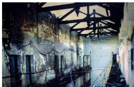
Figure 4: Interior damage to Fremantle Prison's main cell block after the riot in 1988
