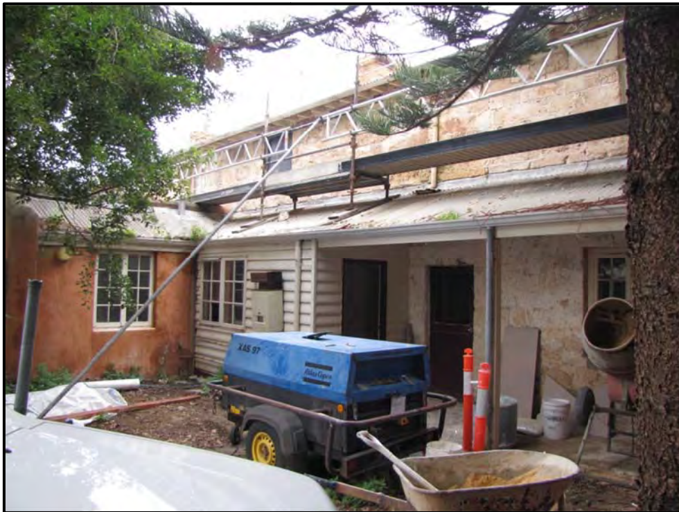
Plate 3: View of W of rear yard and façade of cottage, block W2, house 35/37
